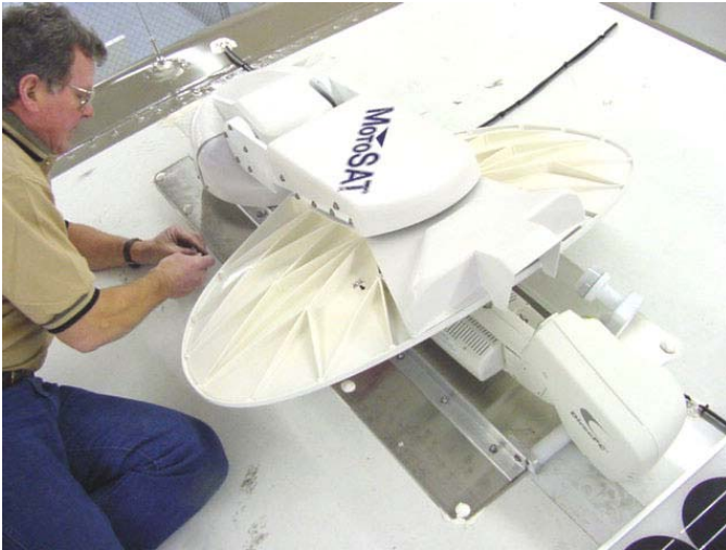
Connect cables to dish mount to complete the install on top of roof.
