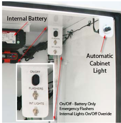
An onboard battery powers cabinet lights and the trailer's emergency flashes when the generator is not running. Helpful for dark nights.
